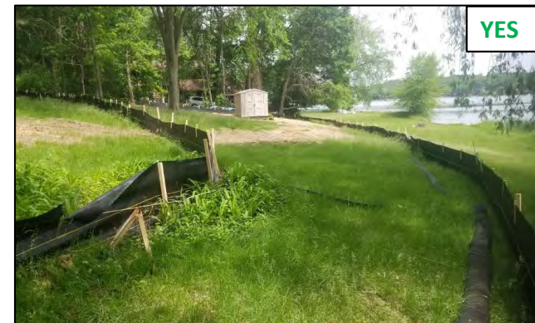
Double layer of silt fence with grass buffer next to Big Marine Lake.
